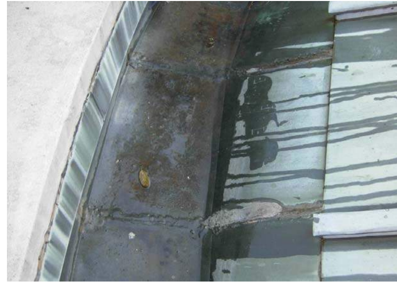
Image 9: Two improperly soldered flat lock seams, both with attempted re-soldering and/or sealant patch. These are in radius built in gutter areas "C", thus close transverse seams.
