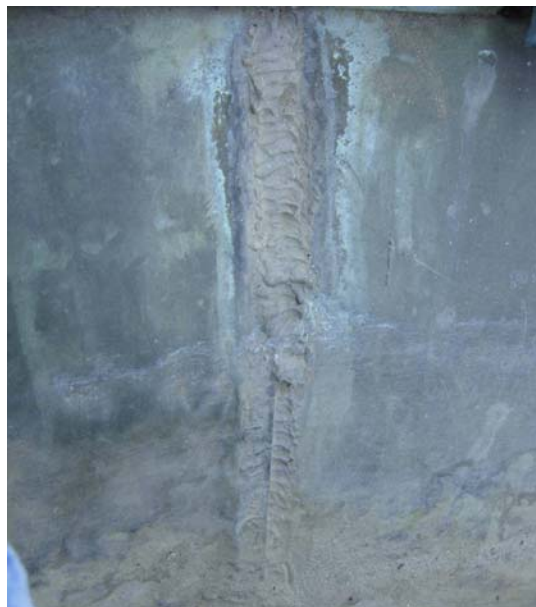
Image 8: Improperly soldered flat lock seam. Lower portion was original; upper appears to represent an attempted re-soldering of a failed seam.
