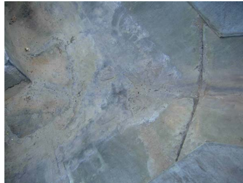
Image 10: improperly soldered flat lock seams, lap seams, and patches at corner roof area "B" North
