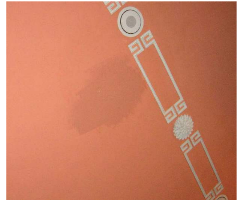
Image 5: Ceiling central portion under roof area "B"— area of prior plaster damage repainted
