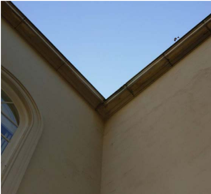
Image 1: Fascia/Soffit Water damage corresponding to downspout, valley, scupper roof area "B" North
