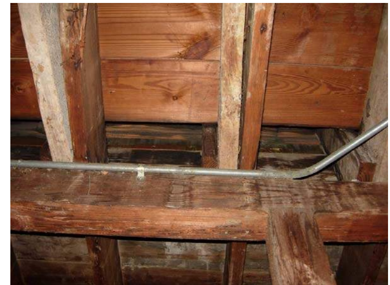
Image 6: Evidence of water infiltration under low slope roof ventilator
