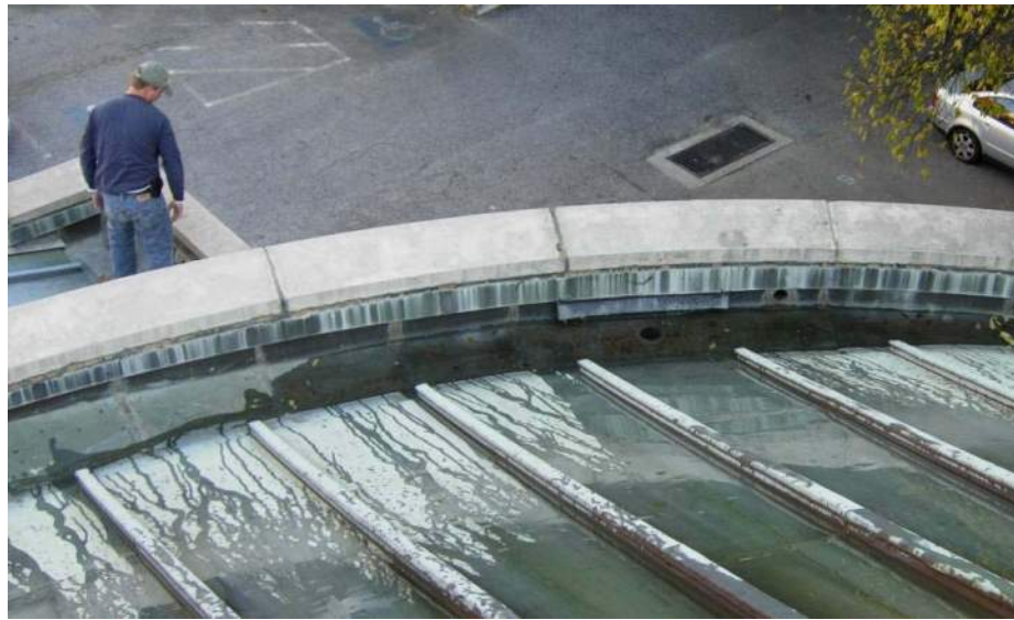
Image 7: Water test in gutter section "C" South, showing clogged drain, also excess copper piece under flashing
