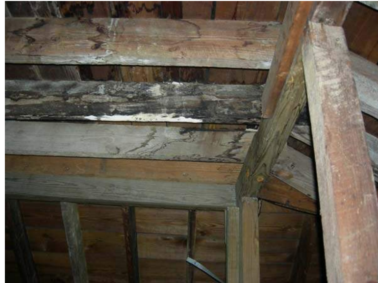
Photograph 04 Water damage at roof rafters
